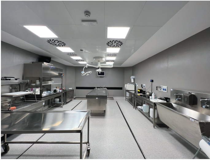
Photo: BSL3 autopsy facility. From the first author's personal collection. Used with permission.
